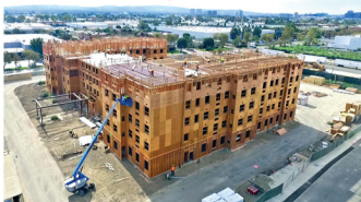
Work is well underway on a 5-story, 168-room Staybridge Suites Extended Stay Hotel that Meridian is constructing in Irvine, California.
